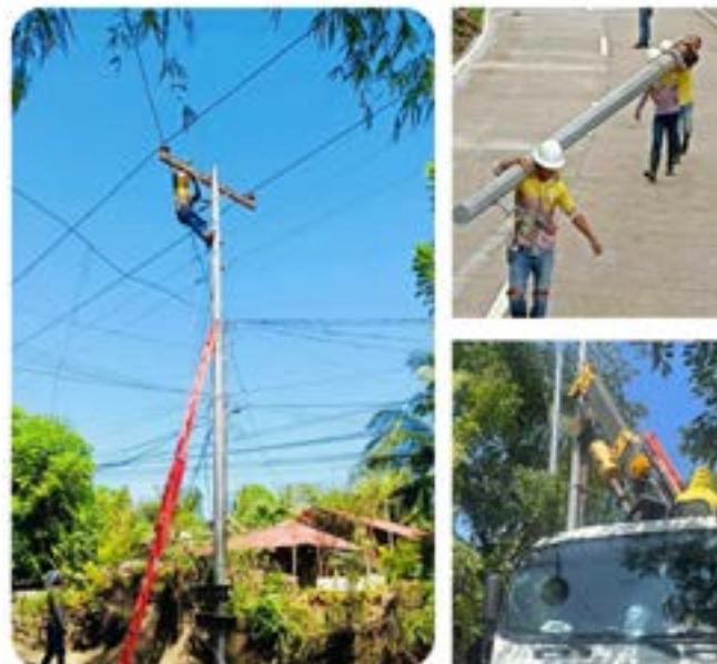
Warriors of Lights facilitating conversion of lines from bare to tree wires and replacement of poles
